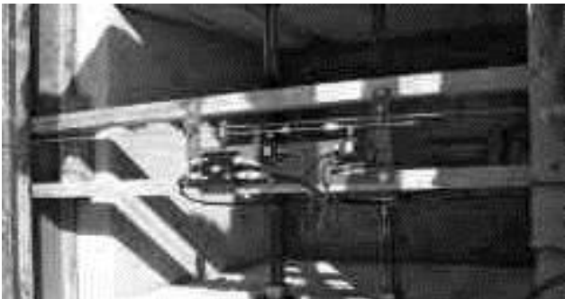
Electrical monitoring device
